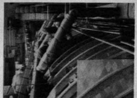
Also backstage, plumbing and insulation are put in place for a working model.
